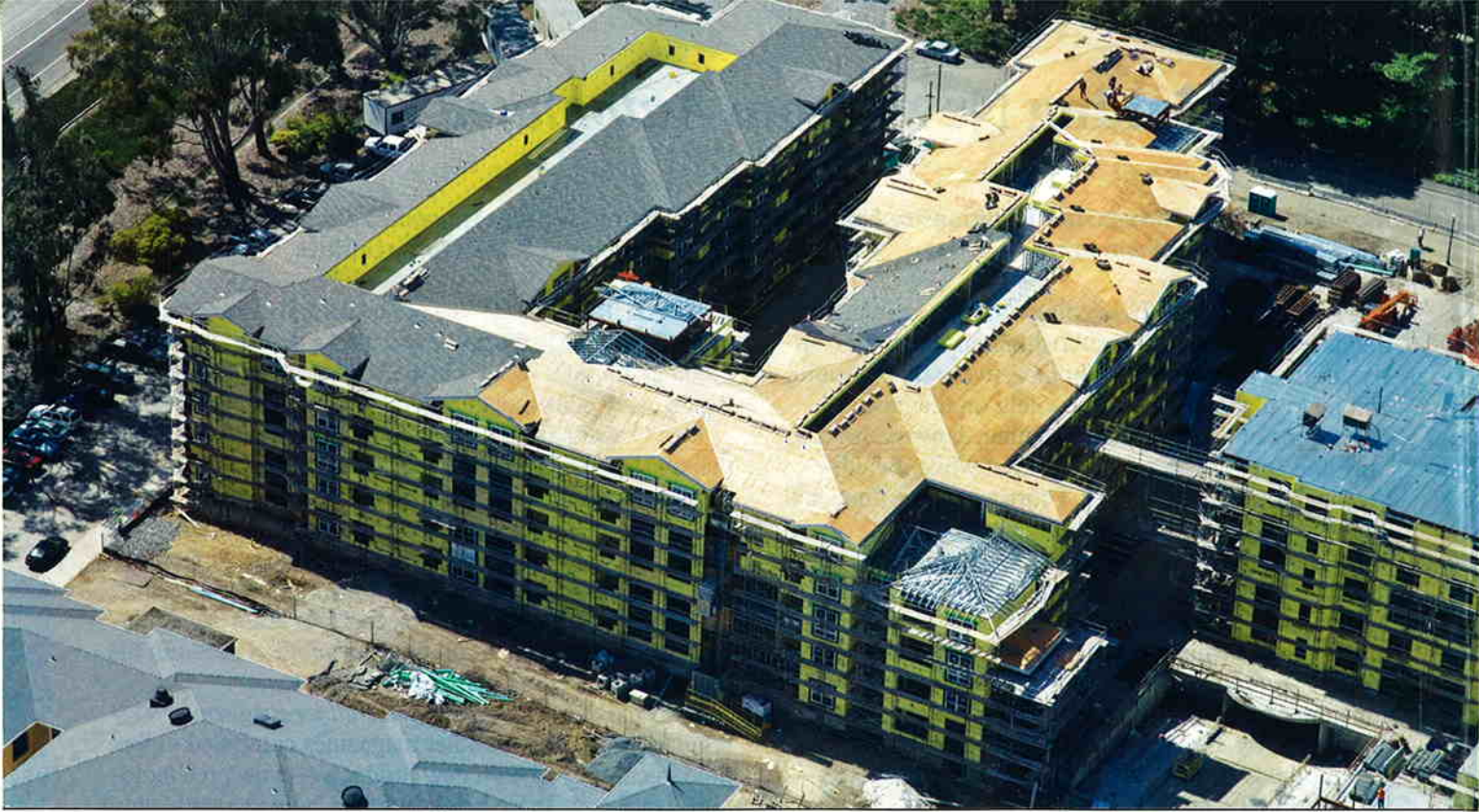
The Crossing in San Bruno, CA with cold-formed steel trusses for a retail and multi-family complex near the San Francisco airport. Team Panels hopes to expand beyond its Colorado facility to offer the same fast, solid construction opportunities across the nation.
