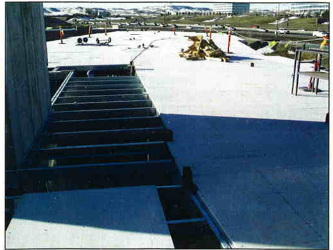
High-strength Fortacrete structural panels also were used in the Candlewood Suites project for the flooring applications.
