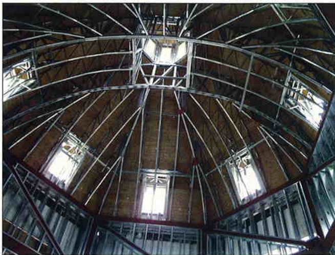
Looking up inside the steel truss section at the dome for a retail center built with Team Panels at Walnut Creek near Broomfield, CO.
