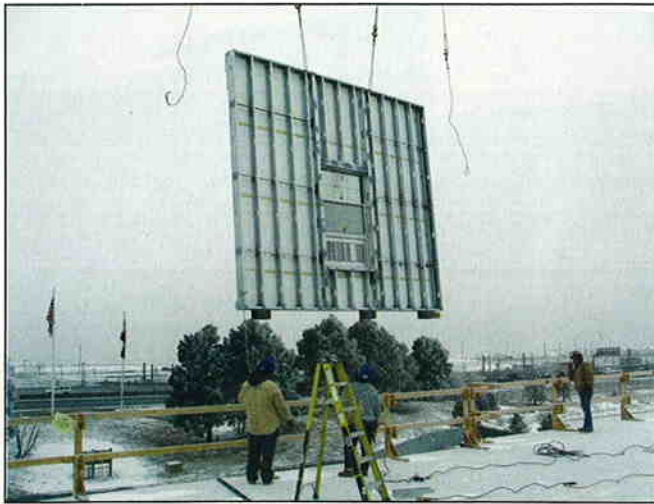
A panel is lowered into place at The Candlewood Suites-Meridian Business Park in south Denver, CO. Team Panels pays extra attention to every component's details so installation teams have faster set-ups.
