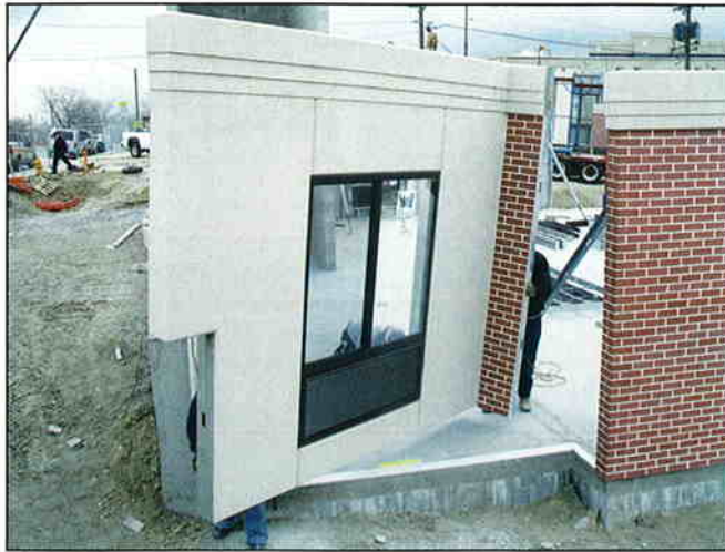
At The Hampton Inn in Denver, CO. Team Panels used prefinished panels (shown) with windows installed and floor panels and trusses erected in a small, challenging construction site.
