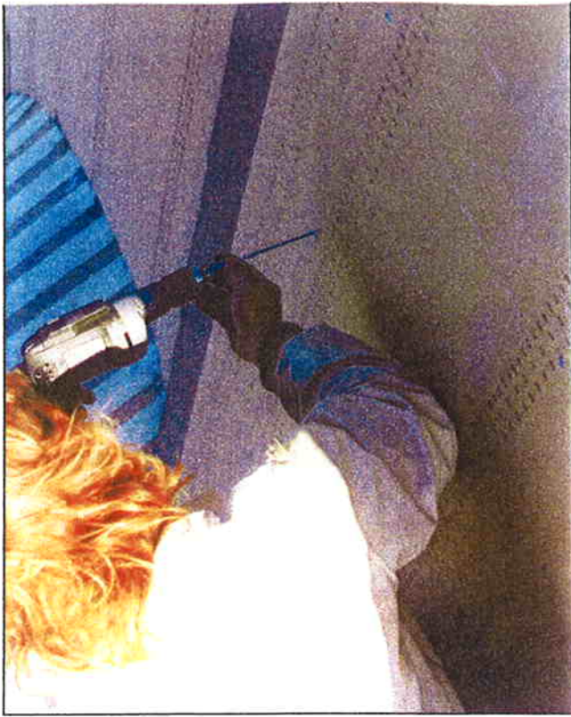
Installation of long screws in a highly insulated roof deck assembly. If a roofing assembly or its parts fail to satisfy applicable code requirements, the architect can potentially be held liable.
