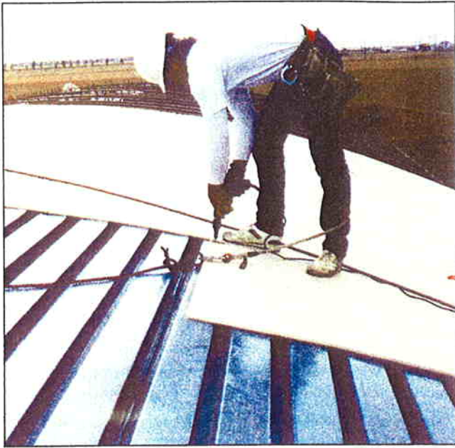
This worker fastens the roofing substrate board to a curved steel deck surface prior to installation of standing seam metal roof covering. Under IBC and ASCE 7, more stringent standards now apply to different sections of a roofing assembly.
